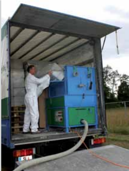
An assistant fills the injection machine on the truck with the ISOCELL cellulose insulation.
